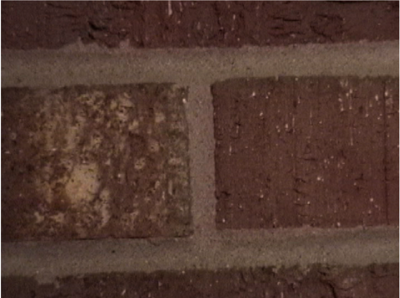
Figure 1: Uncompressed Raw Data (TIFF) Crack to be measured at the border of the brick/mortar interface. at center of the field of view.
